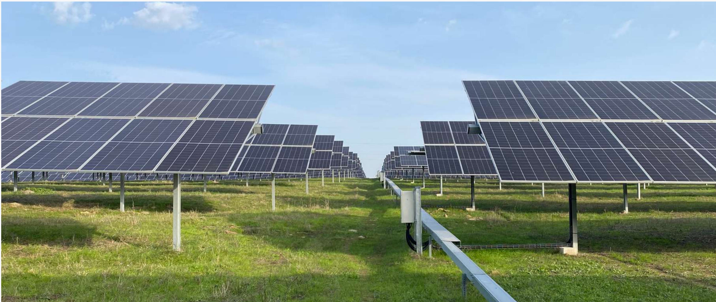
Olivenza Solar Plant
