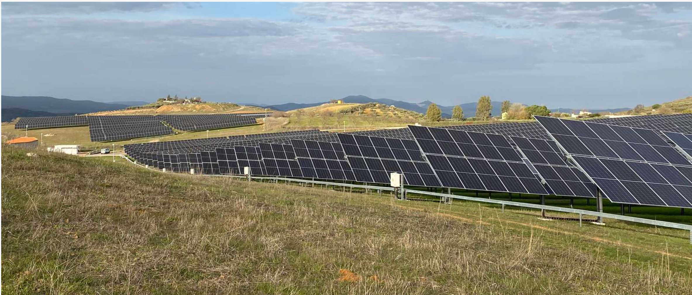
Zafra PV Solar Plant
